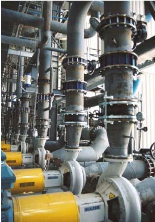
Center Line ® RS installed in a thin juice station
